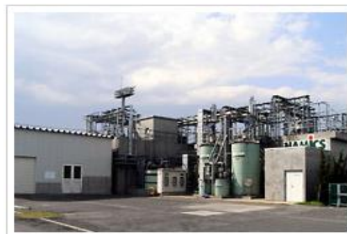
Wastewater treatment facilities (Head Office/Factory)
