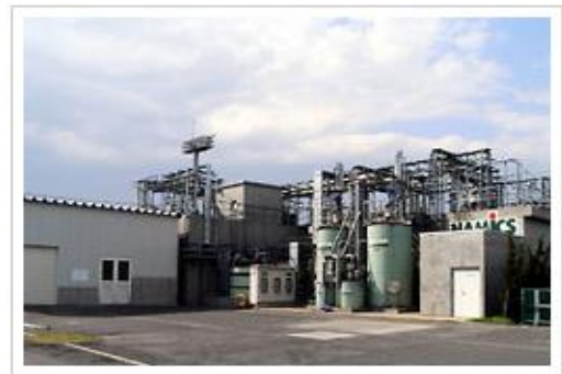
Wastewater treatment facilities (Head Office/Factory)
